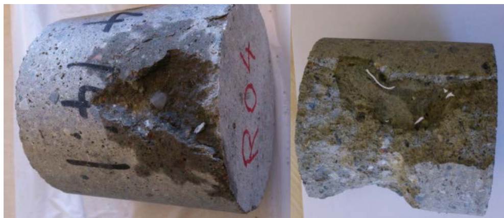
Figure 3. Water repellent effect on two drilled cores. On the left, a reference specimen showing the dark wet interior, and on the right, one with the hydrophobic admixture where there is not such a visible contrast. Both specimens had a 0.4 w/c-ratio.
