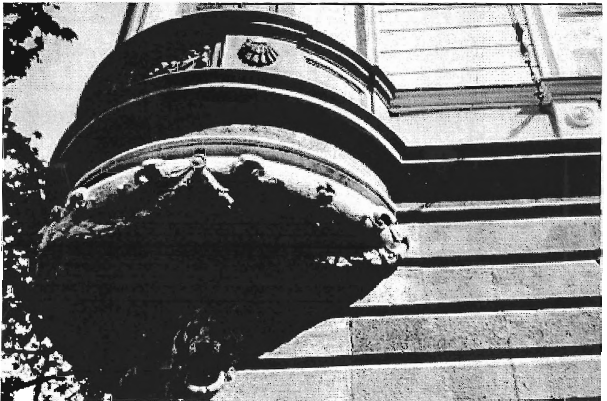
PHOTO 9 A special way of using our Hungarian polyurethane treatment for different kind of materials on the same facade (e.g. fixing the deteriorated plaster, stone and brick construction etc.,) by capilair transport from the polyurethane through the seperated layer and fixing to the brick wall behind.
