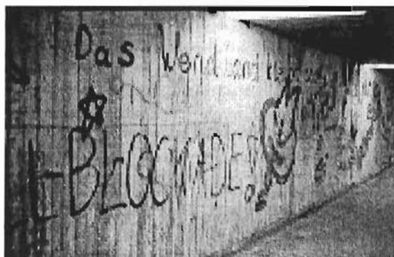
PHOTO 2 Graffiti on concrete
